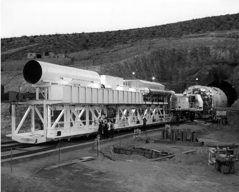
Figure 17.3 Tunnel boring machine begins excavation at Yucca Mountain. Source: US Department of Energy.
