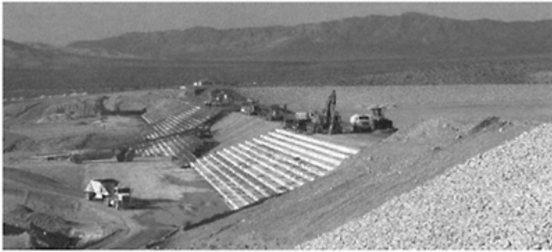
Figure 1. Stepped overflow protection system for a detention basin in west Las Vegas under construction (Courtesy of M.R. DELCAU and USACE-LA District).
