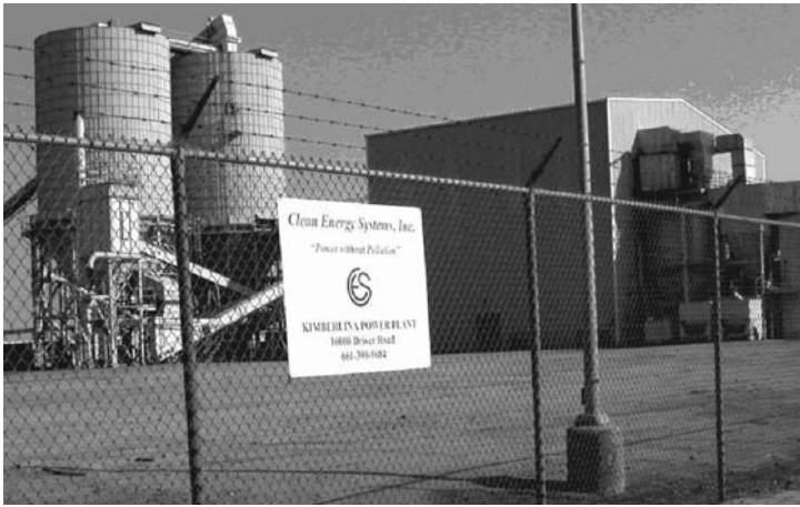
FIGURE 2.5 First in the world ZEPP of 5 MW in Kimberlina, California, put in operation in March 2005 by CES with the cycle in Figure 2.4 ( http://www.cleanenergysystems.com/technology.html ).
