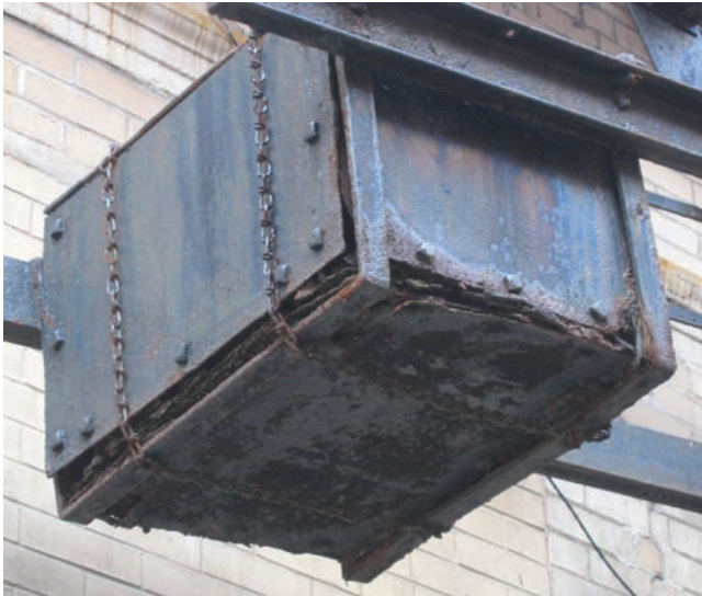
FIGURE 4.21 A box with distinct macro characteristics of exfoliation corrosion.
