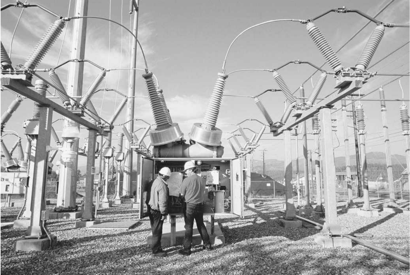
Pend Oreille Utility District workers at a control box in a power substation. (Corbis-Bettmann)
