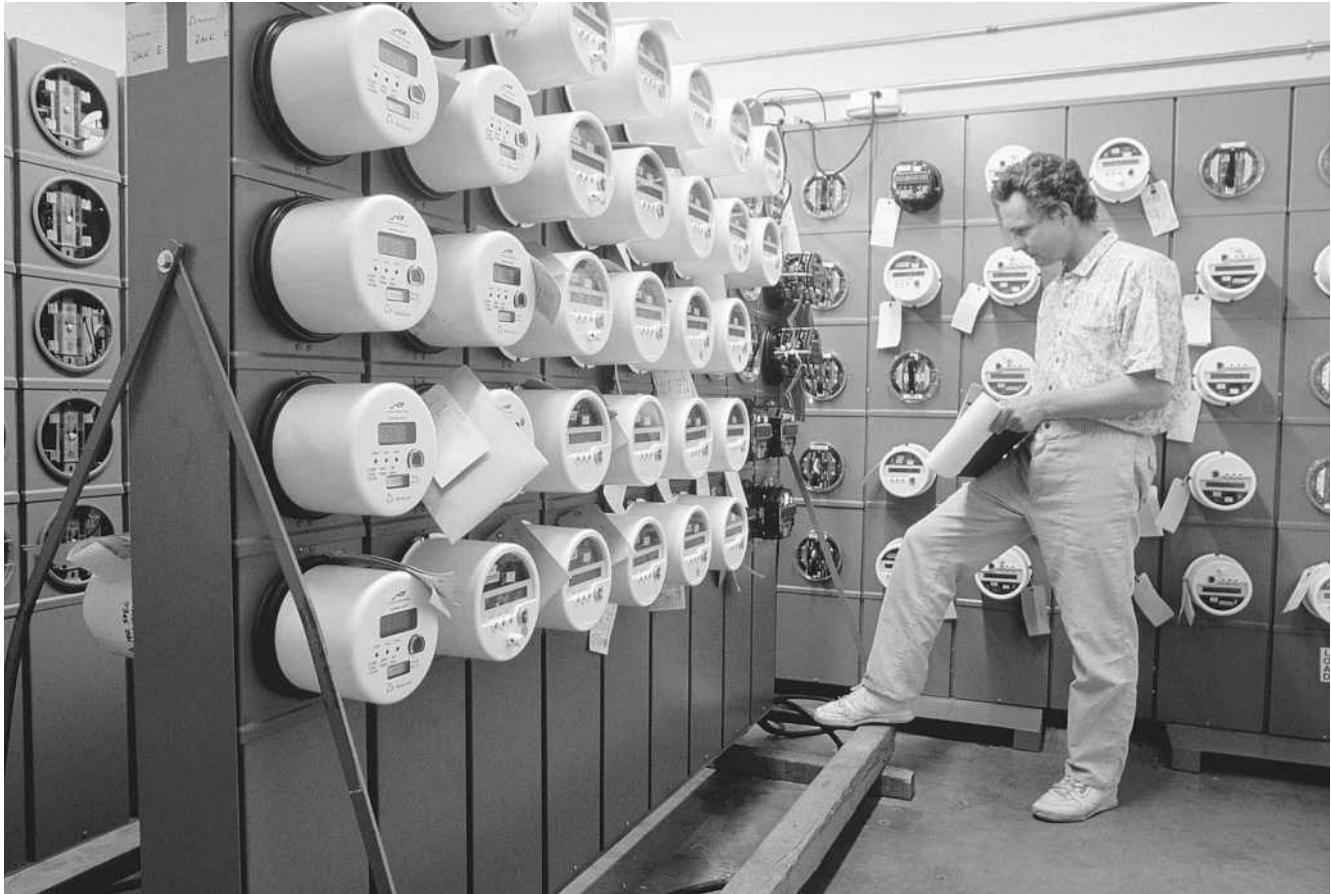
A Southern California Edison employee logs test results at the company's electric meter site. (Corbis-Bettmann)
