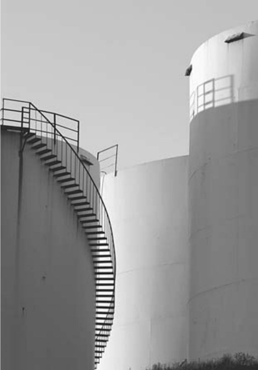
FIGURE 3.4 Outside aboveground storage tanks
