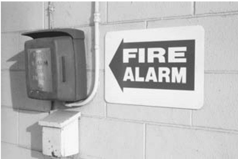
FIGURE 8.1 Fire alarm pull station
