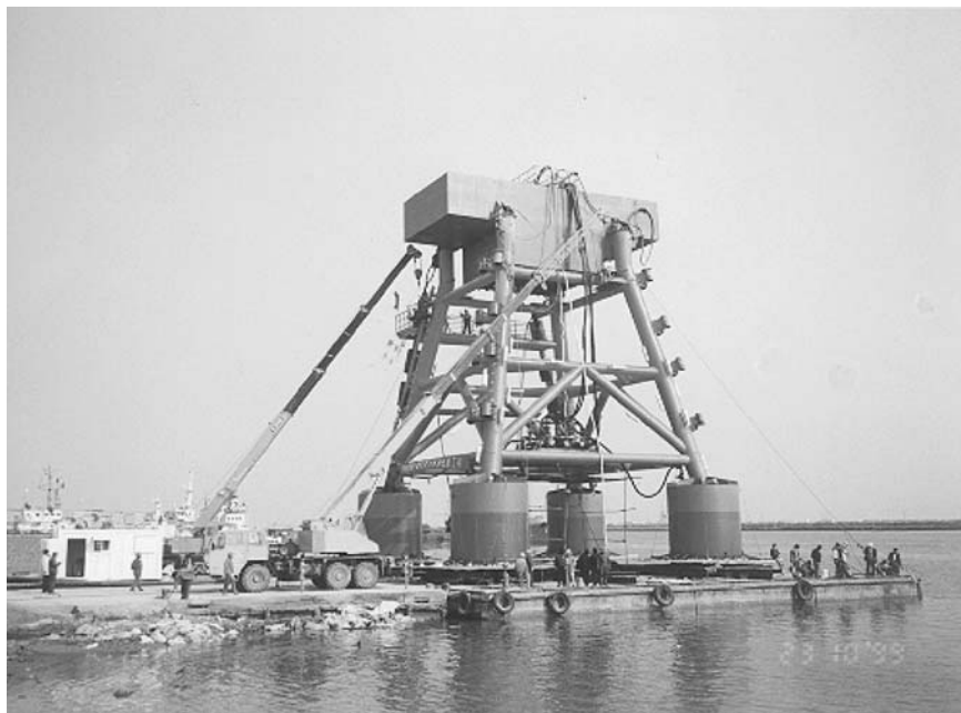
Figure 14.14 Bucket foundation with deck frames of the CB20B platform erected on the dock. The T-shaped structure on the top is the 4-compartment water tank
