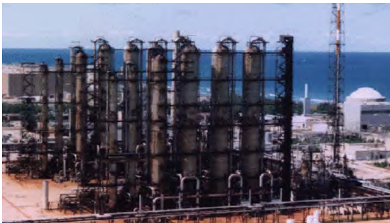
Fig. 8.14 Aerial view of the Bruce D 2 O plant (now decommissioned) ( www.sno.phy.queensu.ca/sno )
