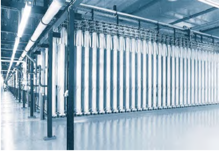
Fig. 8.11 Separation hall with centrifuges at the Gronau Enrichment Plant, Germany (Photo credit. www.urenco.com )
