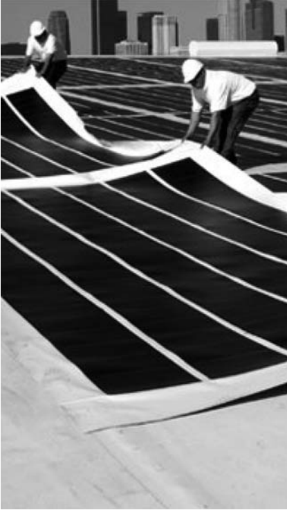
Figure 1.33 Easy installation by Solar Integrated of a lightweight white single-ply roofing membrane, and thin-film photovoltaic membrane transforms commercial and industrial roofs in clean energy generators. (Source. Solar Integrated).
