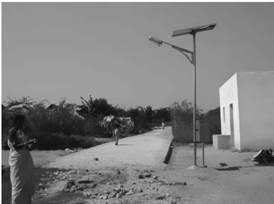
Figure 2.21 Street lighting installed in 2006 in the roads of Maharashtra, India, uses PV to power LED lamps at night. (Photo courtesy of Grameen Surya Bijlee Foundation, www.suryabijlee.com ).
