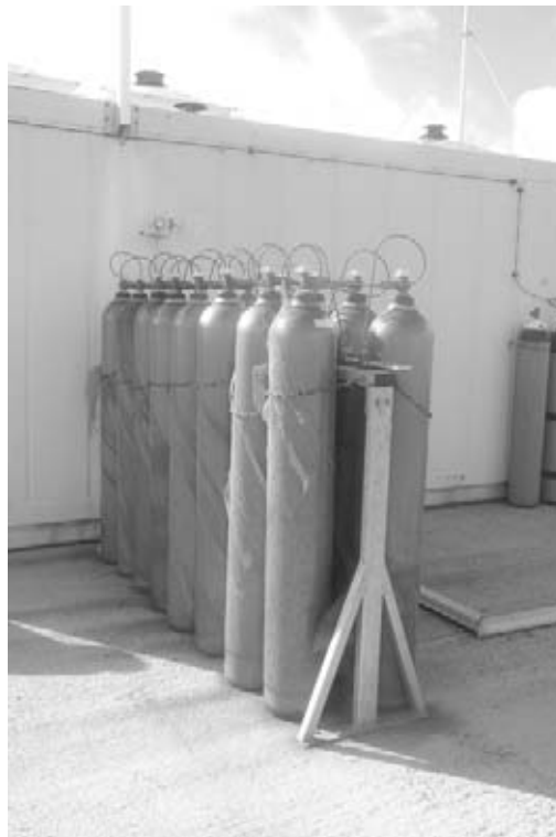
Figure 4-24 Compressed hydrogen storage at the PURE Energy Centre.
