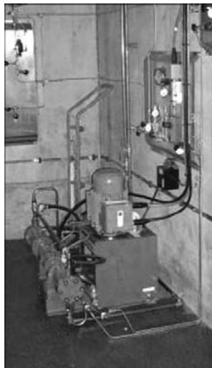
Figure 4-25 Hydrogen compressor at HARI project, West Beacon Farm. Image courtesy Dr Rupert Gammon.
