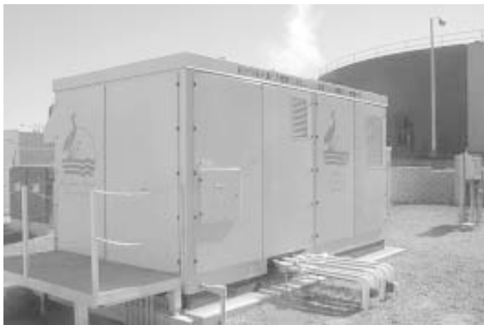
6.11 Anaerobic digester gas (ADG) fuels this PureCell™ fuel cell powerplant at a wastewater treatment plant in Yonkers, New York. Image Courtesy of: UTC Power Corporation.
