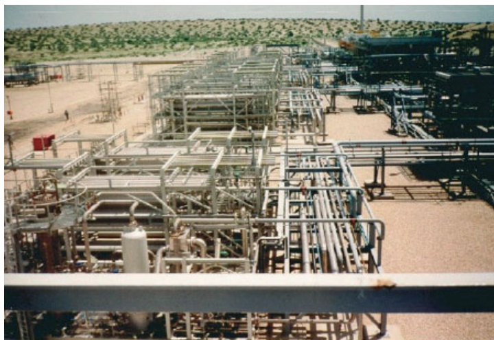
Figure 8.10 Photograph of the 500-million scfd CO 2 removal plant installed by UOP at Kandawari, Pakistan. The UOP Separex system reduces CO 2 content of a natural-gas stream from 6.5 to 2% CO 2 . Photo used courtesy of UOP, LLC.
