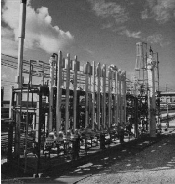
Figure 8.8 Photograph of a Permea hydrogen recovery unit installed at an ammonia plant. The hollow fiber modules are mounted vertically [6].
