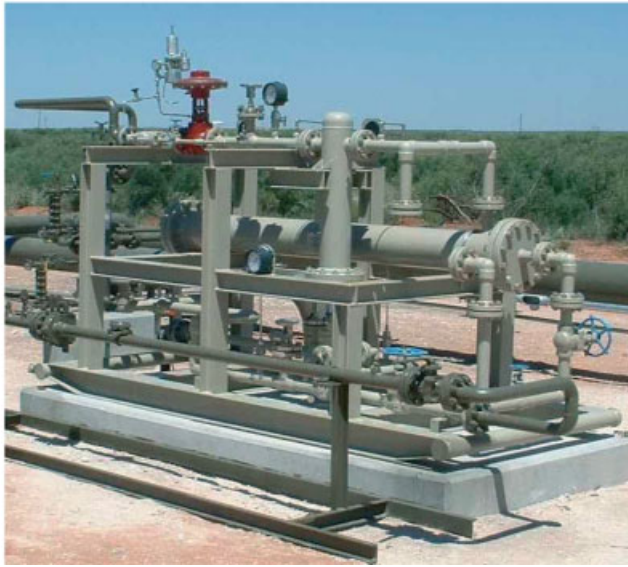
Figure 8.12 Block diagram and photograph of a membrane fuel-gas conditioning unit (FGCU) used for a field gas compressor engine (the unit uses silicone rubber membranes in spiral-wound modules). The membrane modules are contained in the horizontal pressure vessels. The unit produces 0.5–1.0 MMscfd of clean gas. Reproduced with permission from Ind. Eng. Chem. Res. 2008, 47(7), 2109–2121. Copyright 2008 American Chemical Society [17].
