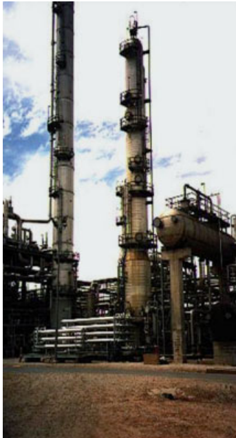
Figure 7.4 Air Liquide/Medal membrane unit replacement of amine scrubbing towers (used with permission).
