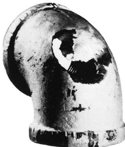
Figure 17.20 Impingement failure of an elbow that was part of a steam condensate line. (Photograph courtesy of Mars G. Fontana. From M. G. Fontana, Corrosion Engineering , 3rd edition. Copyright © 1986 by McGraw-Hill Book Company. Reproduced with permission.)
