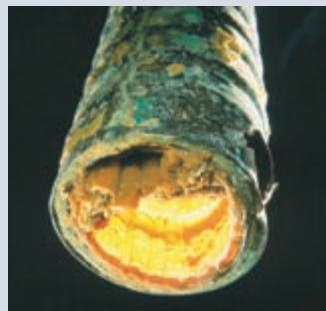
◀ Figure 18.18 A section of water pipe that has been coated on the inside with \text{CaCO}_3 and other insoluble salts deposited from hard water.
