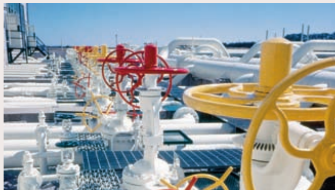
▲ Figure 10.15 A natural gas pipeline relay station.
