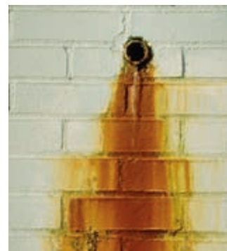
► Figure 23.29 The presence of dissolved iron salts in a water supply leads to stains from deposits of \text{Fe}_2\text{O}_3 .
