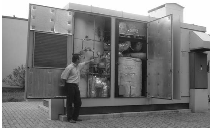
Fig. 2. Fuel cell installed at the public bath of Halle
