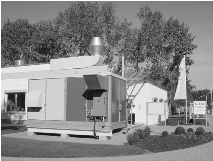
Fig. 3. Installation at Celanese Ventures, in Frankfurt
