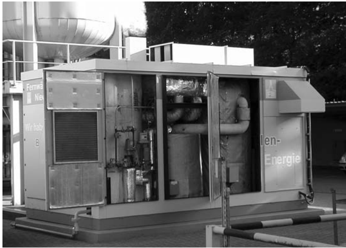
Fig. 6. PC25C fuel cell in Dinslaken, after overhaul
