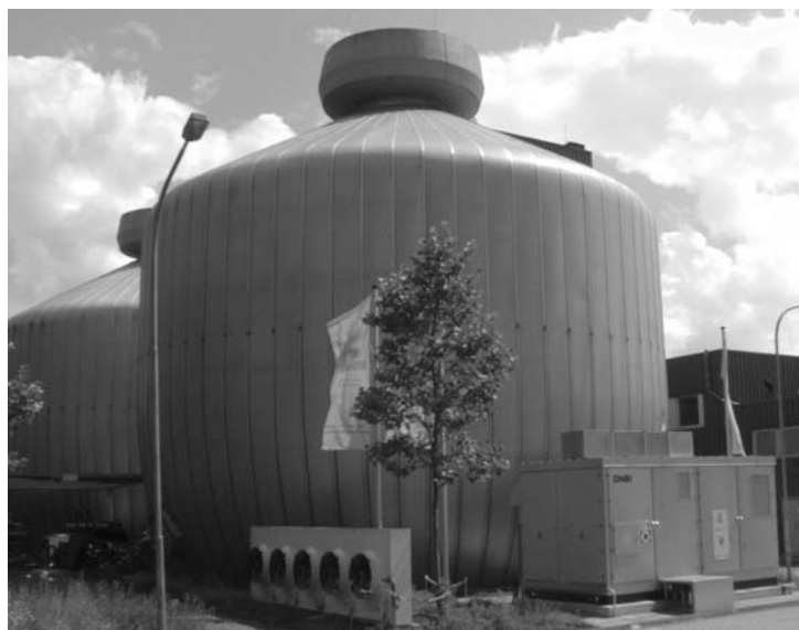
Fig. 4. Fuel cell-anaerobic digester integrated system in Cologne
