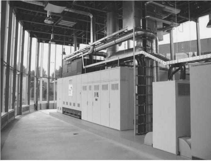
FIGURE 8.4 100-kW SOFC CHP plant of Siemens–Westinghouse in The Netherlands. (Courtesy of Siemens AG, Energy Sector.)
