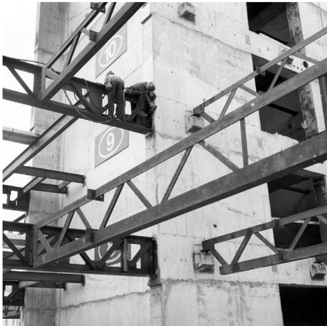
Figure 12.1-17 Floor trusses are typically mechanically fastened to the vertical structure of modern skyscrapers using high-strength bolts and nuts, such as those shown here in the Quaker Tower, Chicago, IL. (Courtesy of Bechtel Corporation, San Francisco, CA, with permission.)
