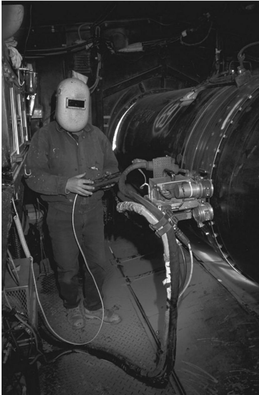
Figure 12.1-14 Joining is essential to the routine scheduled maintenance and unscheduled emergency repair, not only the construction, of nuclear power plant components; it sometimes demands that welding, for example, be done using either mechanized systems operated by welders outside of radioactive areas or by remotely controlled robots within such areas. (Courtesy of Bechtel Corporation, San Francisco, CA, with permission.)
