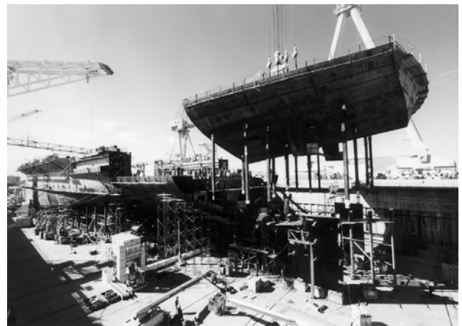
Figure 12.1-20 Ships of all kinds are fabricated by welding small parts into large parts, large parts into structural modules, and modules to one another to construct the hull and superstructure. Here, a larger pre-fabricated modular section of the hull of the carrier USS Reagan is shown being lifted into place for welding to the rest of the hull. (Courtesy of Northrop Grumman Corporation’s Newport News Shipbuilding, Newport News, VA, with permission.)
