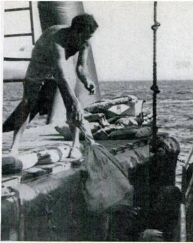
CHUCK HIGGINS drops bag of mix from platform. On bottom, divers place bags between feeder pipes
