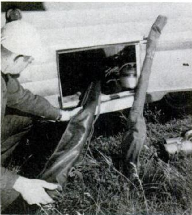
SABRE-SAW OPENING; add flanges, bin door from trailer supply to make an outside-access storage box
