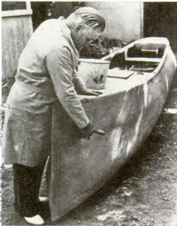
Crushed rock compound applied over wire mesh forms the thin but sturdy walls of this 26-foot boat
