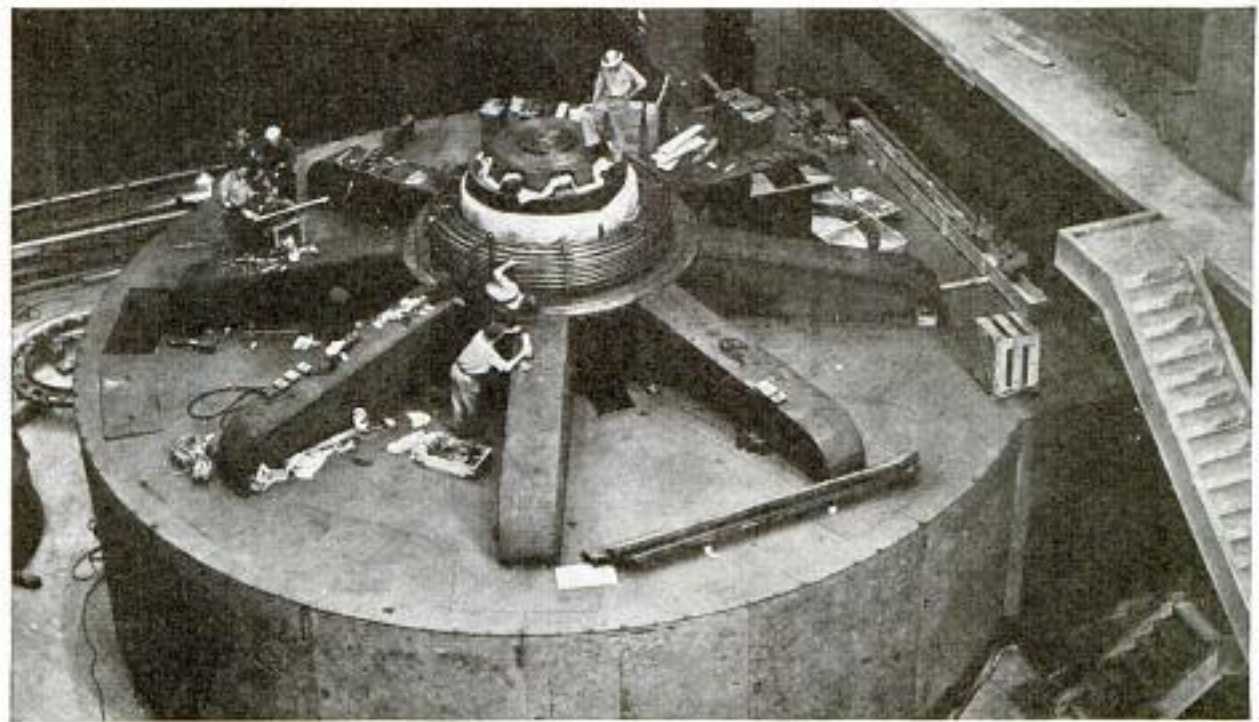
Installing the first giant water-wheel generator at Grand Coulee dam, which delivers 108,000 kilowatts
