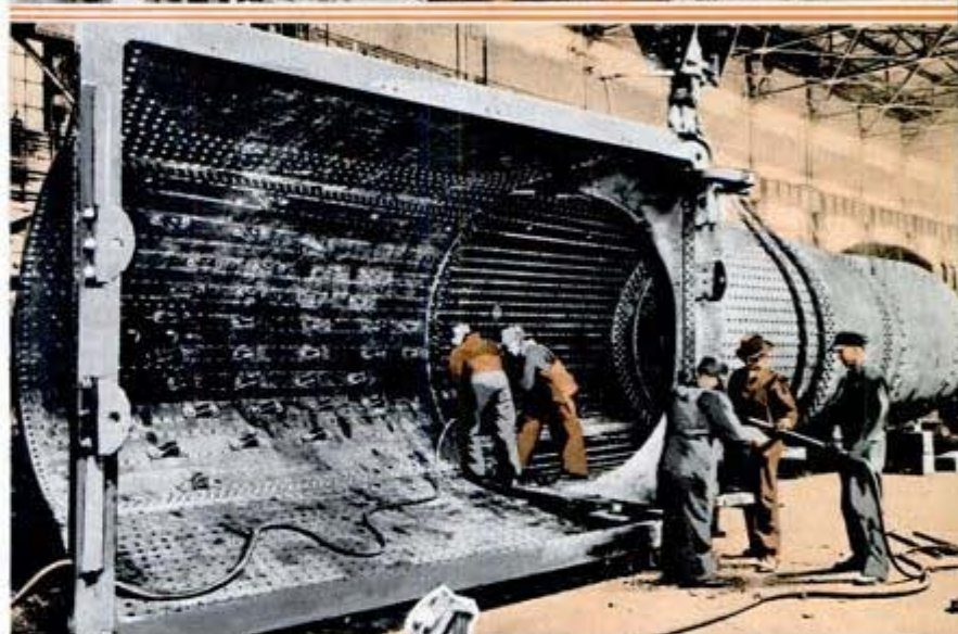
Top, Pennsylvania engineer gets orders by radio from caboose in experimental installation. Center, building a big Norfolk & Western locomotive
