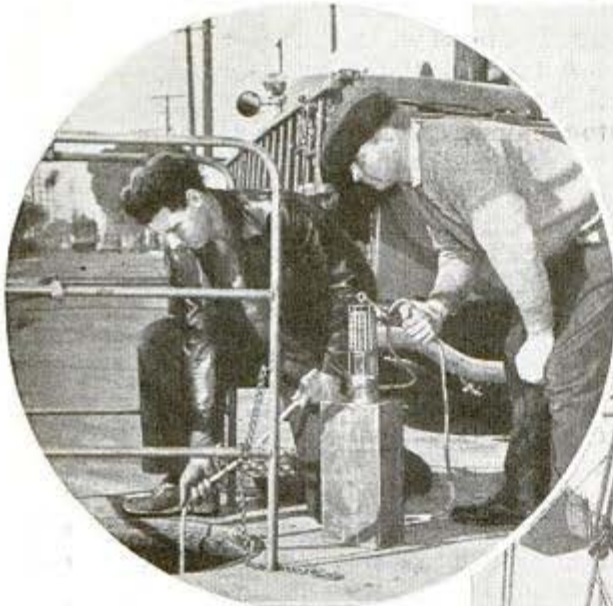
Before they go down to repair damaged electric conduits, workmen test the manhole for carbon dioxide gas
