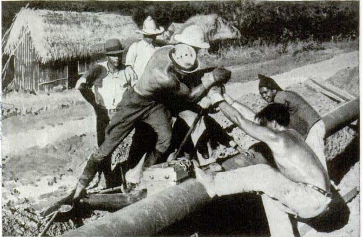
Here is a pipe bender in operation. Deep in the jungle, where remoteness and hopeless transportation bar heavy machinery, crude tools like these and human muscles become a necessity
