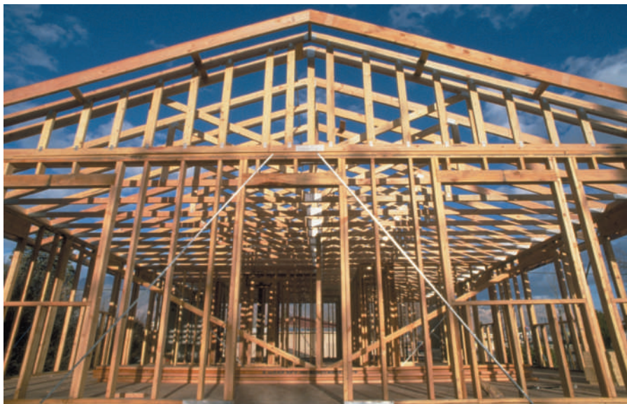
The wood frame of a new house being erected in Lone Pine, California.
